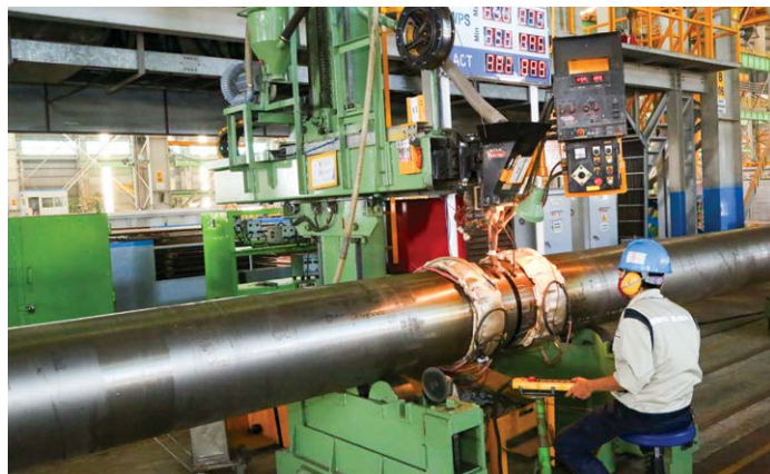
Welder welds a Butt-Joint Pipe to Pipe for a Platen Super Heater Outlet Manifold with Visualization of the AMP's displayed on an electronic board
