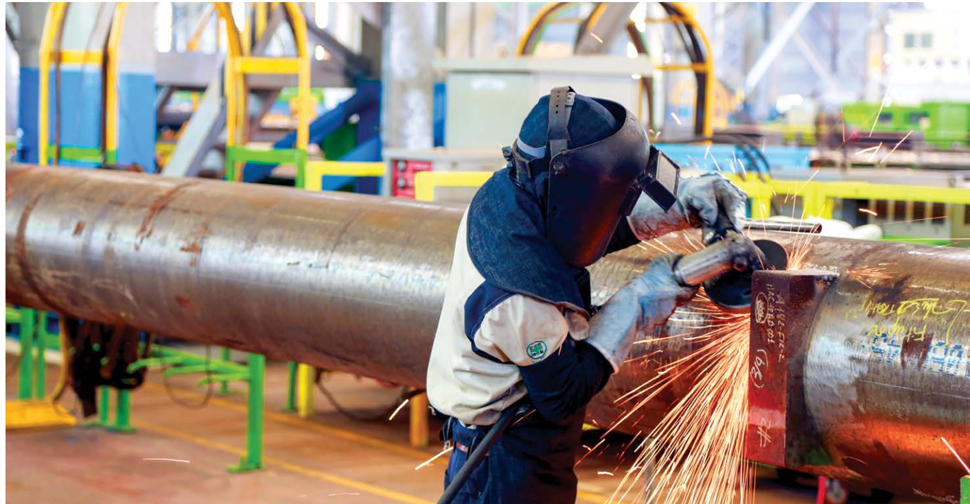
A Boiler worker grinds a Primary Reheater Inlet Header for the Vinh Tan 4 Thermal Power Plant Project
