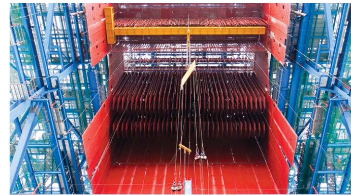
Erection of Platen Super Heater and Final Super Heater at the Mong Duong II Power Plant
