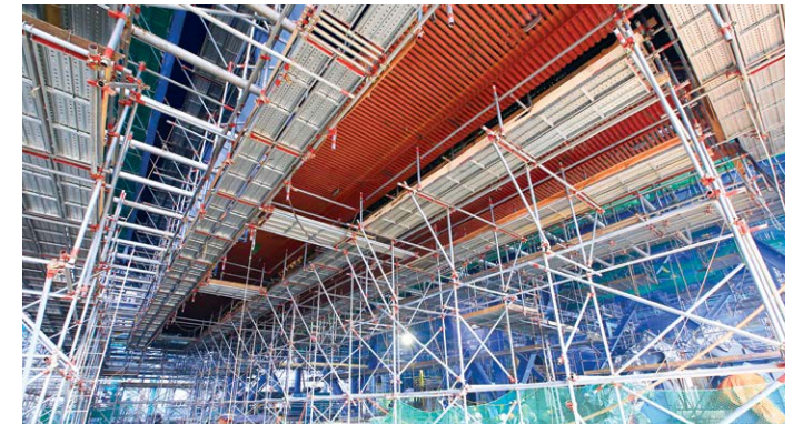
Erection of Spiral Hopper Discharge Wall Panel and Furnace Inlet Header at the Site of the Mong Duong II Power Plant
