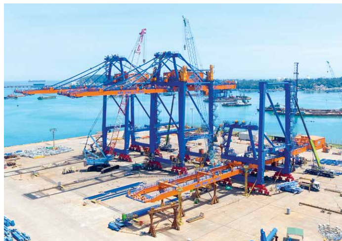
6 units of Panamax cranes under manufacturing for Gemadept Corp., Dinh Vu, Vietnam
