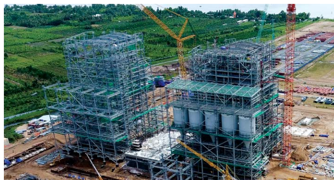
Erecting Steel Structures at the Song Hau I Power Plant Site, Vietnam
