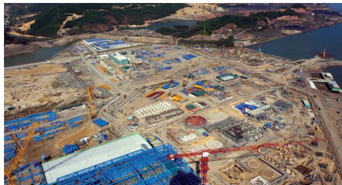
Erecting Steel Structures at the Mong Duong II Power Plant Site, Vietnam
